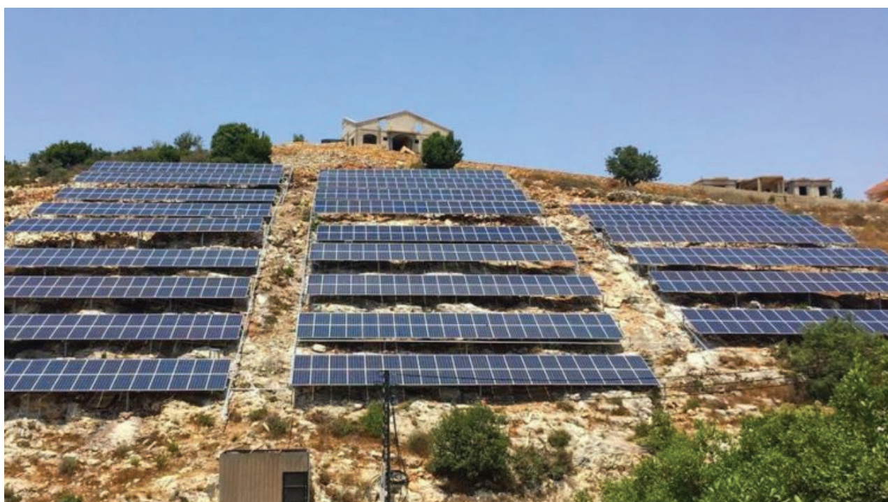
Figure 23: Kabrikha's community solar PV project, South Lebanon
